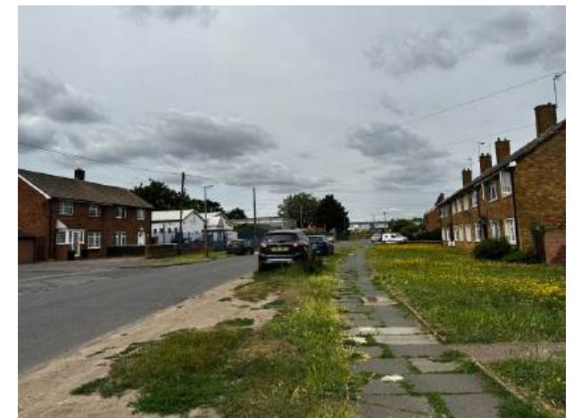
Poor quality footway surfaces cause tripping hazards.
